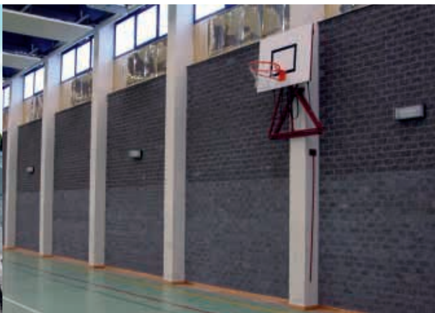
Sports hall in fair-faced acoustic masonry: combination of fine structural blocks and split blocks
